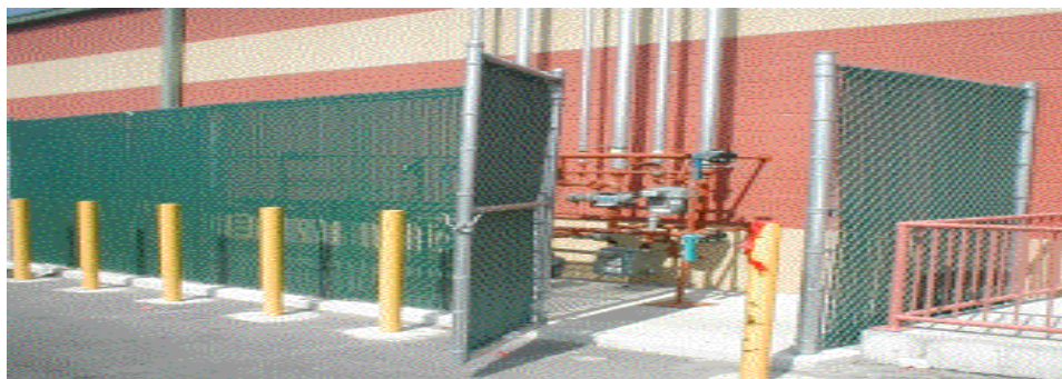
Light Commercial Multi-Metered Installation, Protected By Bollards and Fence. In the rear of Shopping Center Loading Dock.
